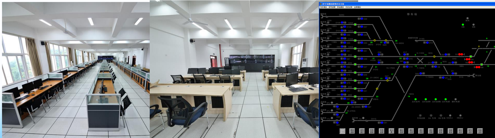
High speed railway dispatch center and Metro Operation control center
