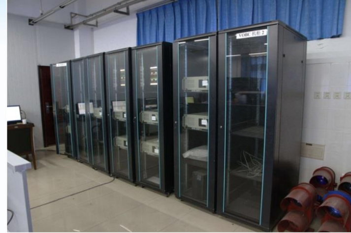
Signaling control testing and verification system
