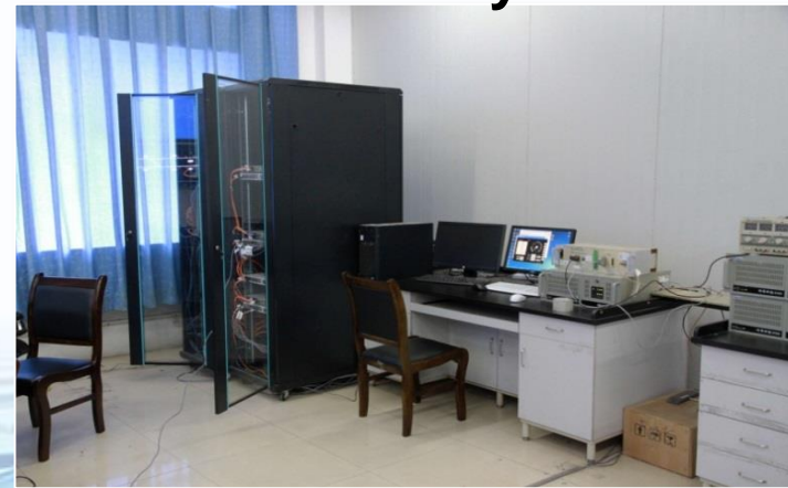
DCS monitoring system
