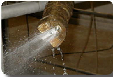
Automatic cleaning nozzle for a redox sensor (CERLIC,ARR)
