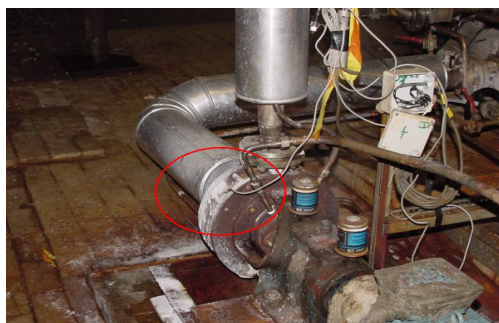
A process temperature probe failure is responsible for burns sustained by a technician during maintenance work (ARIA 30723, Dreal Nord Pas de Calais)
