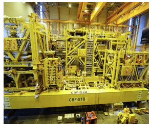
Figure: First compressor train for the Åsgard field (Statoil)
