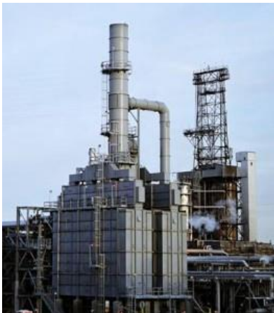
Delayed coker heater
