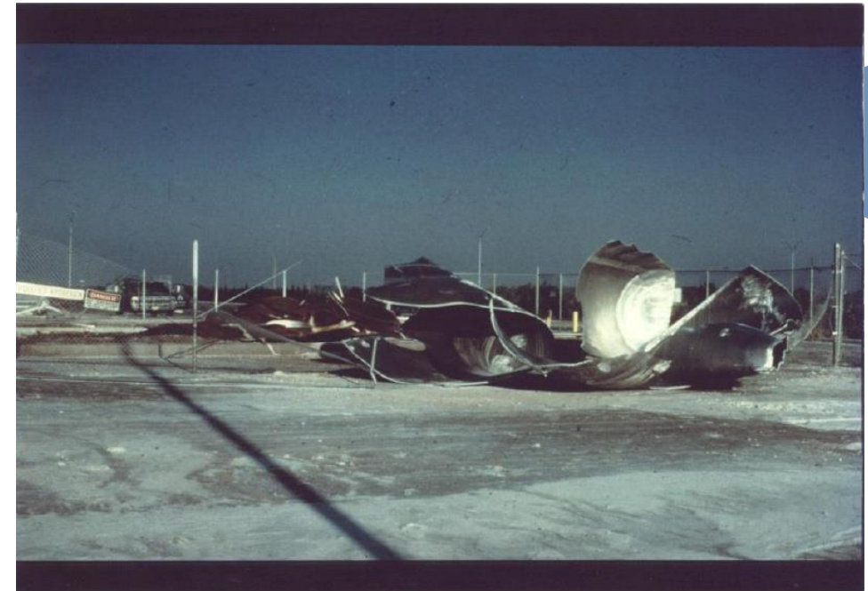
[Feldman et al., “1974 LHY Tank Failure”, SAF75U002 RRS . Air Products internal report (1975)
