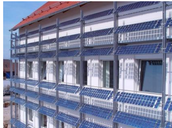
Figure 7. PV shading at Council Building, Edingen, Germany
