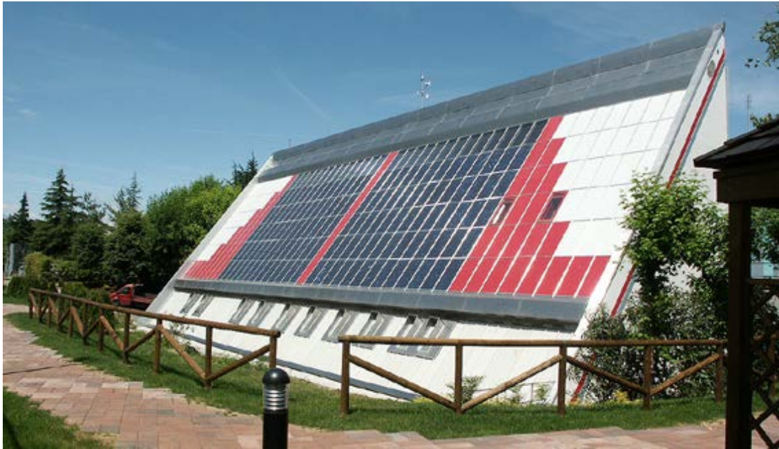
FIG 4.2: PV combined with a thermal system (PVT) façade of Fiat Research Center
