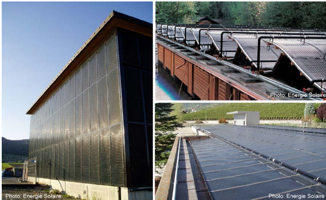
FIG 2.8 (Left) Unglazed flat plate collectors integrated on the façade, (Right top, bottom) Unglazed flat plate collectors integrated on the roof
