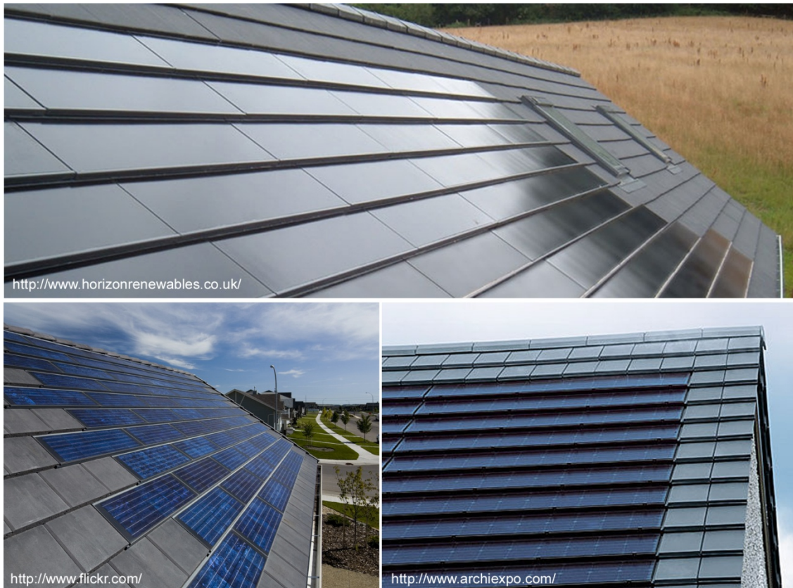
FIG 4.5: Integrated PV roof tiles on the roof
