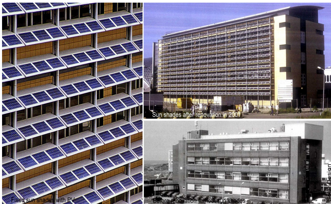
FIG 4.15: PV used as shading in the Energy Research Centre, Netherlands
