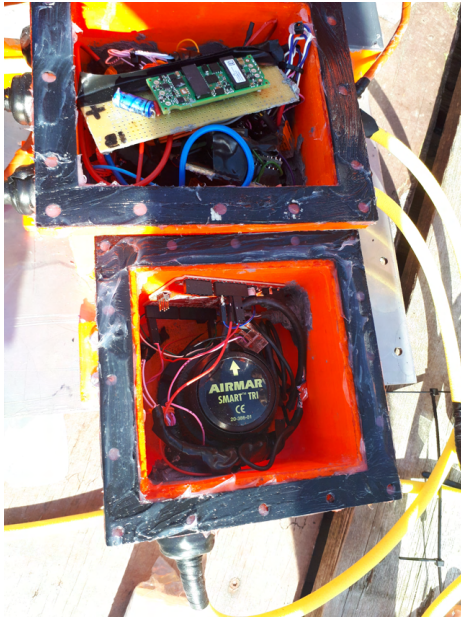
Figure 4.37: Equipment in boxes
