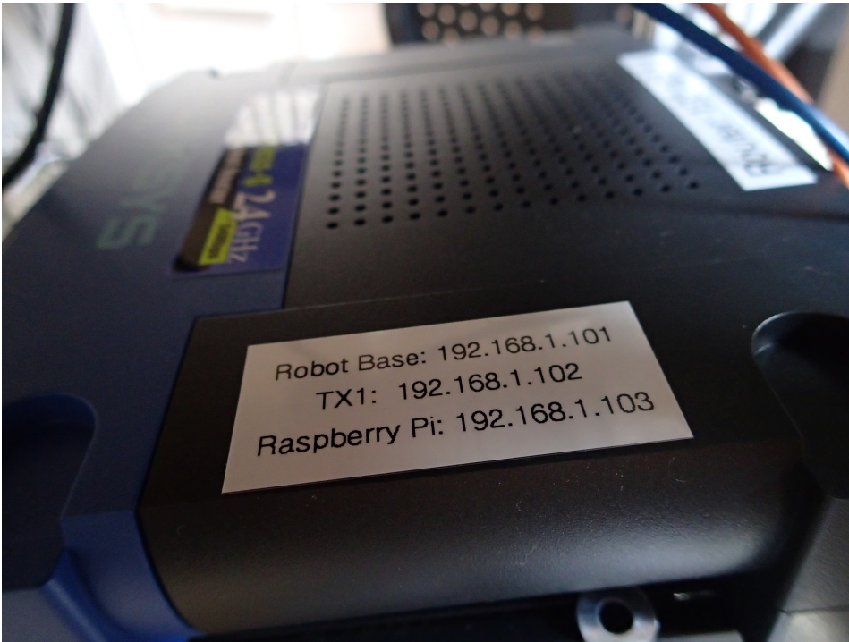
Figure 8.8: I added a label to the router with the current static IPs.
