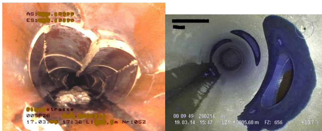
Fig. 1. Damaged sewers and exemplary repairs
