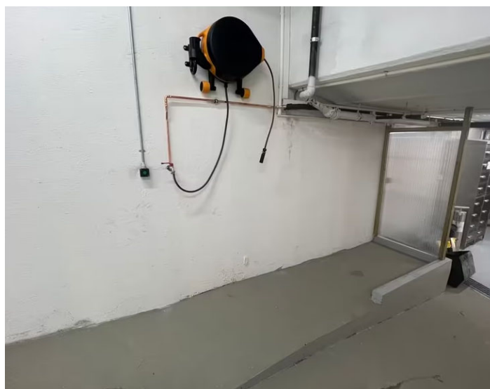
Fig. 1. Bicycle washing stand at Leuthenhaven bicycle hotel, Trondheim
