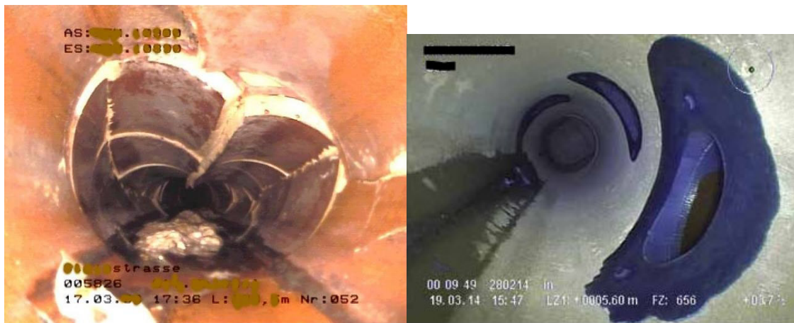
Fig. 1. Damaged sewers and exemplary repairs
