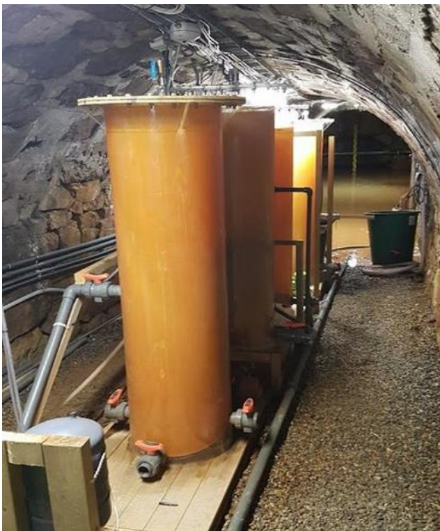
Pilot plant at the field site in Ilsvika
