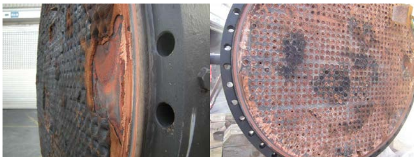
Figure 1: Blocked evaporator pipes
