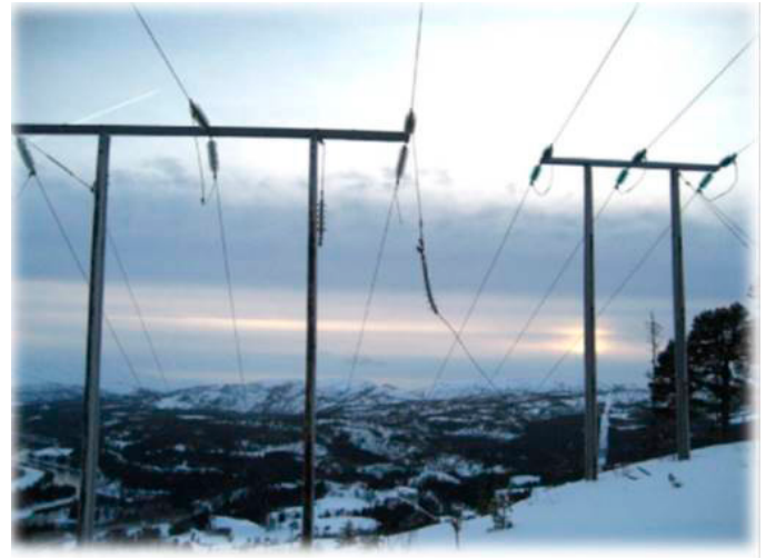
Photograph of conductor fault that caused power oscillations in NTEs network. Taken by technicians in NTE.
