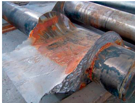
Erosion damage of guide vane
