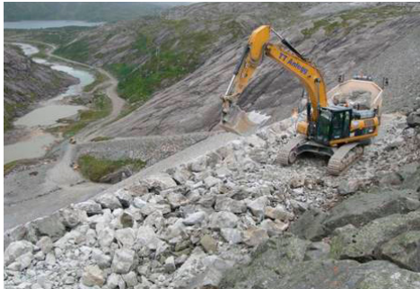
Rehabilitation of Svartevatn dam: placement of riprap stones on the downstream slope
