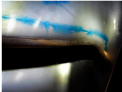
Runner Litjfossen power plant
