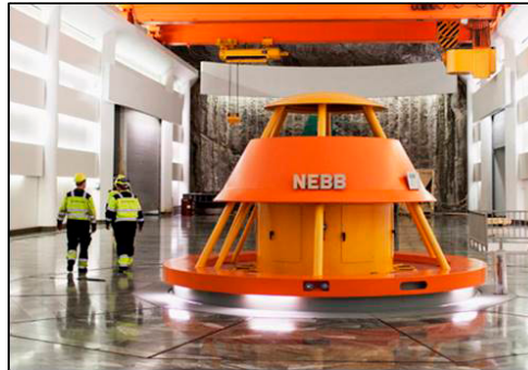
Machine Hall, Tonstad Hydropower Plant
