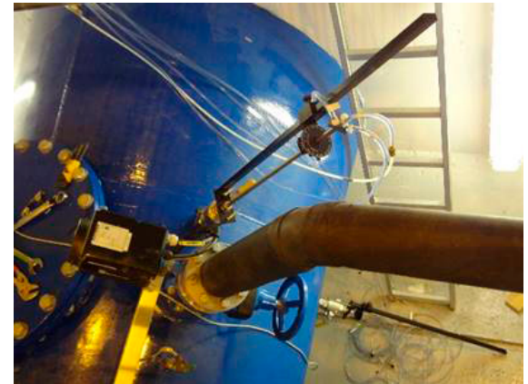
This picture shows two Pitot tubes used to measure the volume flow at Øvre Leirfoss Power Plant.
