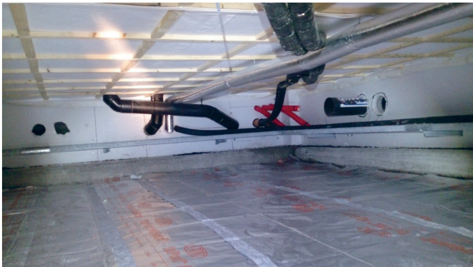
Reflective wind barrier mounted in a crawl space at The ZEB Pilot House Larvik
