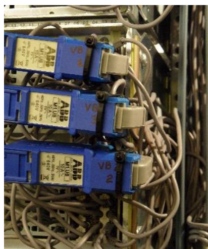
Fig. 4 – Current clamps mounted on current transformers secondary circuit.
