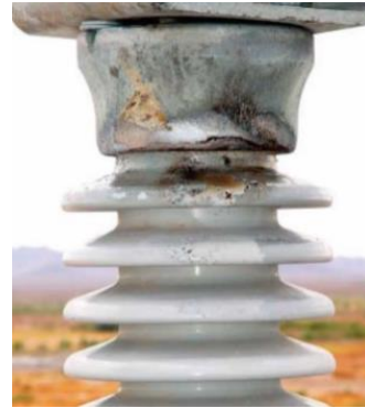
Fig. 3 – Insulator condition post-flashover [2]
