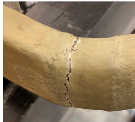
Fig. 6 – Crack in end-winding.
