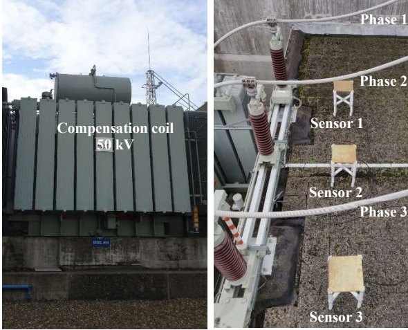
Fig. 2 – Compensation coil (left) and capacitive sensor positioning beneath the overhead lines connecting the compensation coil to the switchgears (right)
