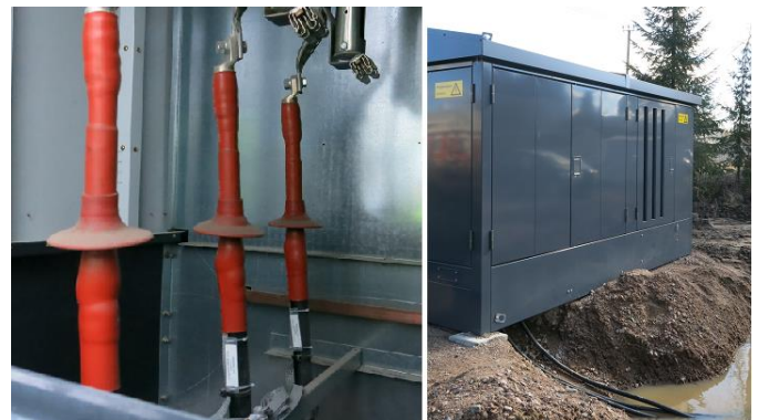
Figure 1. Typical installations sites with dust accumulating on the termination surfaces and water level close to the bottom of the secondary outdoor substation.
