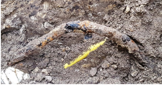
Fig. 13 - Photograph of the damage cable found in the connection monitored in case study 3.
