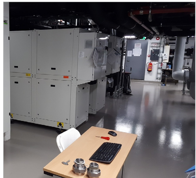
Figure 2. A view of the energy central, seen from the middle of the room. The rather sparsely equipped “work station” hints at the level of automation – necessary human intervention is reduced to a minimum.
