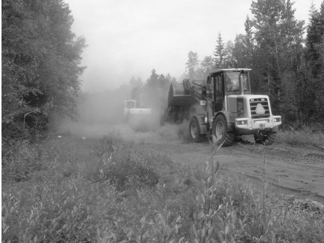
Figure 2: Spreading fly ash from the forest industry on road BD694, Vitåfors, Sweden.
