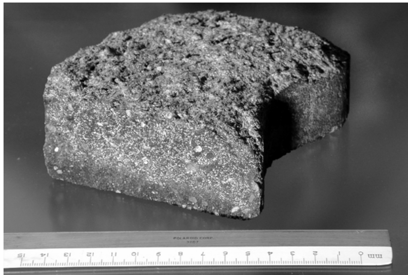
Figure 1: Concrete paving block undergoing sulfate attack.
