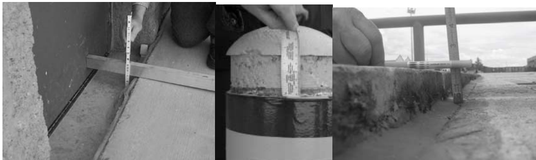
Figure 2: Examples of heaving (from left to right): heaving at door adjacent to maintenance hangar, concrete extruded from a bollard by expansion in recycled concrete base, and heaving of pavement on recycled base adjacent to fuel trench founded on subgrade.
