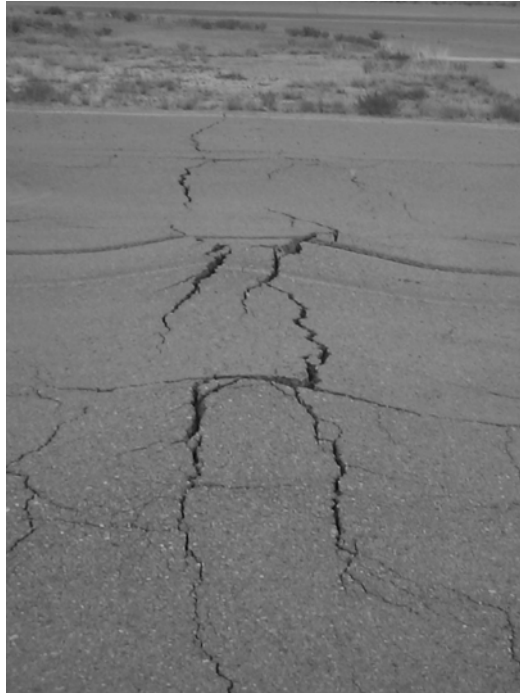
Figure 3: Heaving of a taxiway surface caused by sulfate attack on a cement-stabilized base made with Type V sulfate-resistant cement, Holloman AFB, New Mexico.
