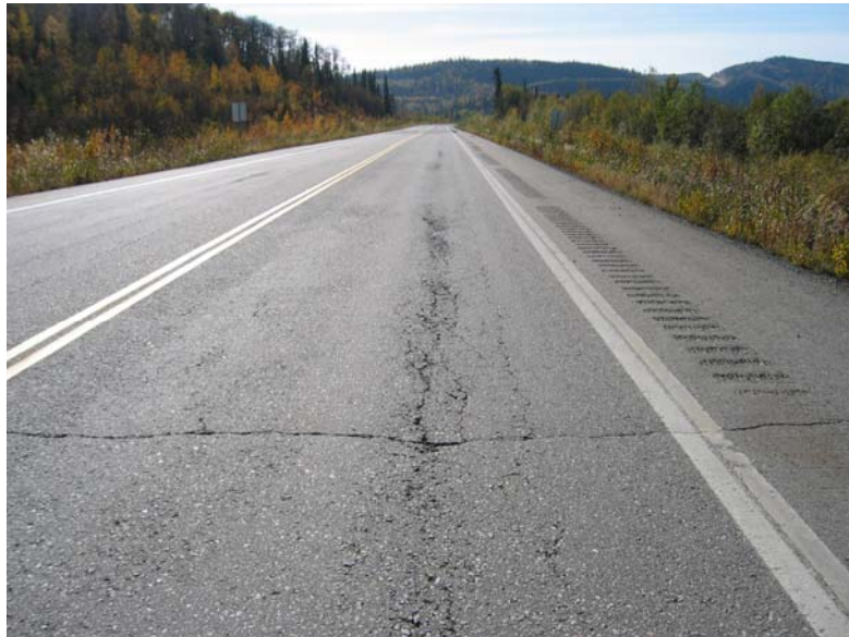
Figure 1: Longitudinal rutting and cracking of a paved road due to thaw weakening of the supporting soil structure. Photo courtesy of Hannele Zubeck.
