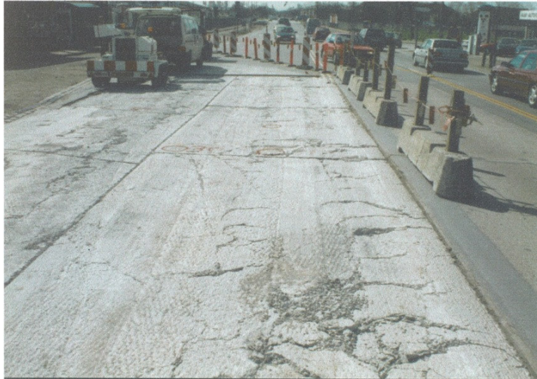
Figure 1: The surface of the crack and seated concrete slabs at the test section
