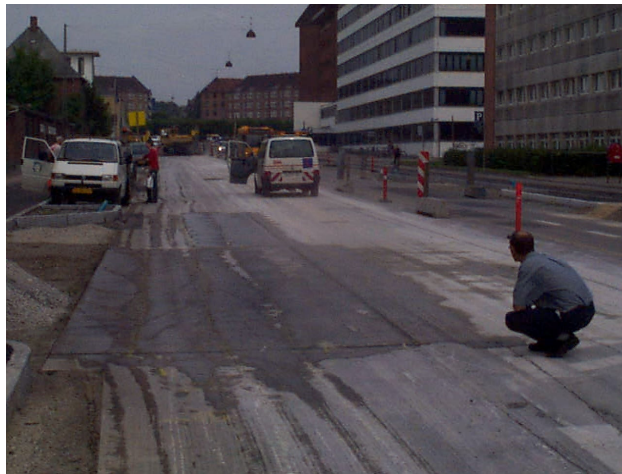
Figure 4: The surface of the cracked and seated surface of the old concrete pavement.
