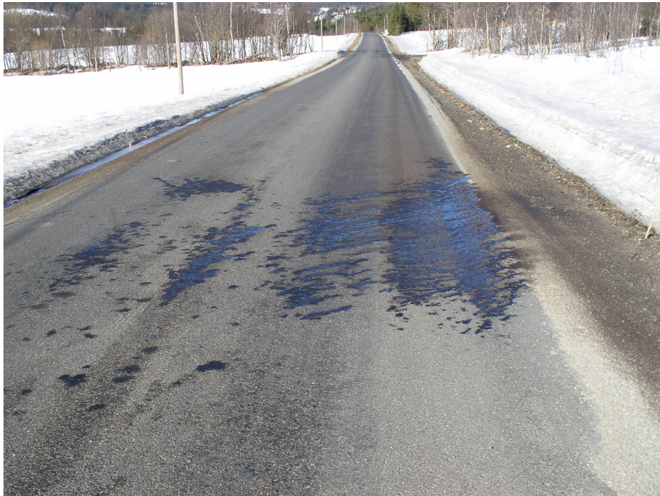
Figure 2: Water pressed through the surface in spring thaw
