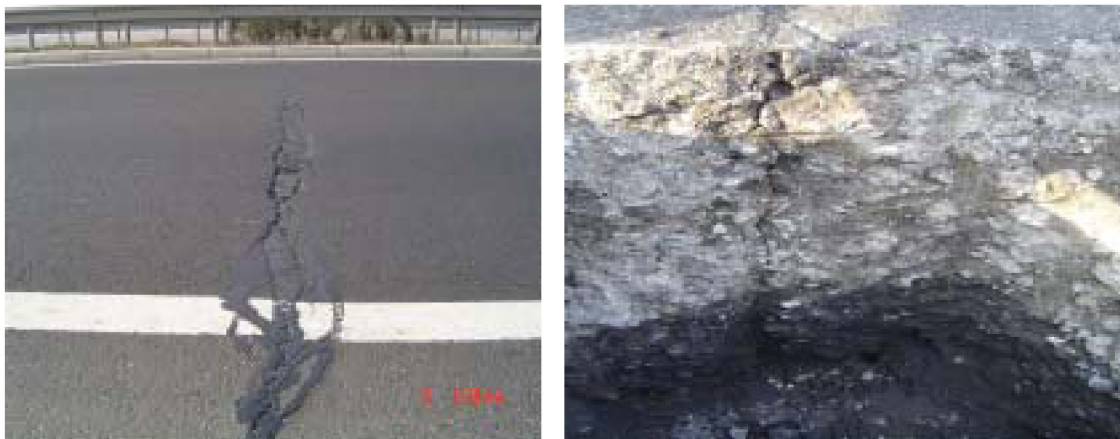
Figure 4: Transverse cracking originating from the hydraulically treated base
