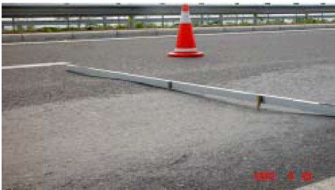
Figure 2: Pavement rutting on Shijiazhuang-Anyang motorway in China
