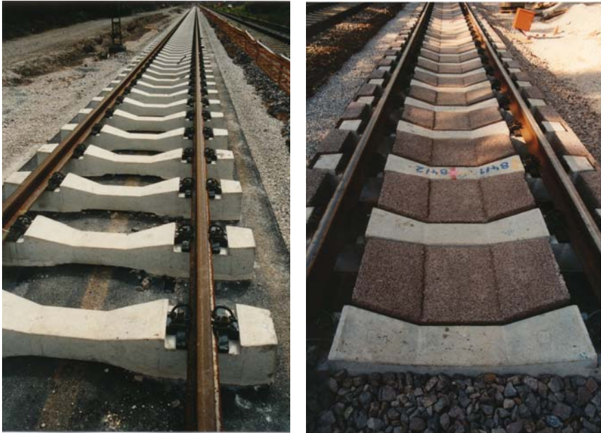
Figure 7: SATO-test section in Waghäusel during construction (left picture) and after installation of prefabricated absorbing elements (wood concrete) or old ballast (bottom of right picture) to reduce noise emission
