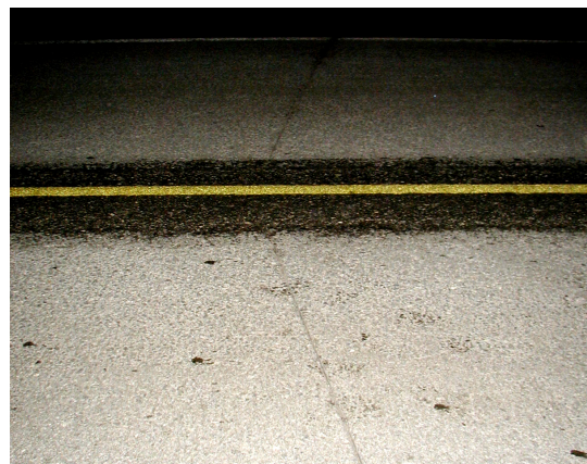
Figure 4: Inclined joints after approximately 15 years service. Longitudinal centre joint was repaired after uncontrolled cracking.
