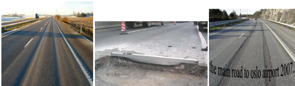
Figure 2: Wheel path rutting (SINTEF web page), rutted pavement cut to show the deformations, and typical studded tire wear (Haugødegård, 2008).
