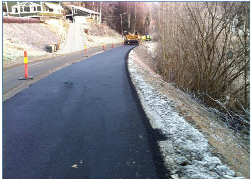
Figure 7: New layer of asphalt. Notice the cogging that is cutted into the untouched part of the road [9] .
