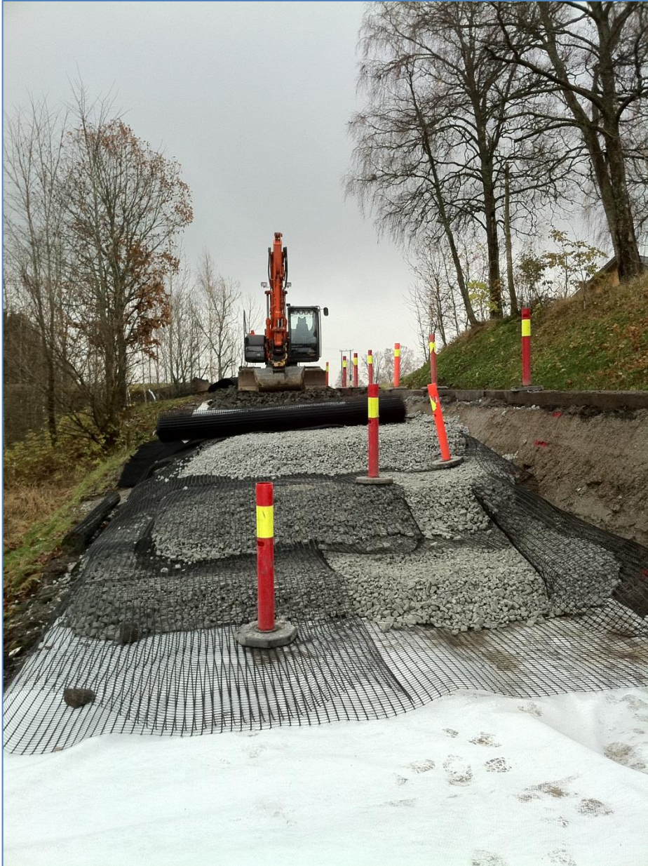
Figure 10: Picture from Fv115 south for Mønster bridge (Østfold, Norway) during constructuin phase. Observe the three layers with foamglass which is separated by reinforcing mesh [9] .
