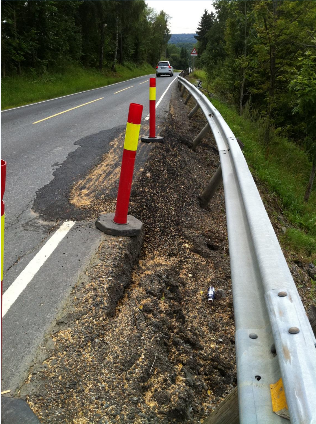
Figure 9: Picture from Fv 115 south for Mønster bridge before the repairations were started in fall 2011 [9] .
