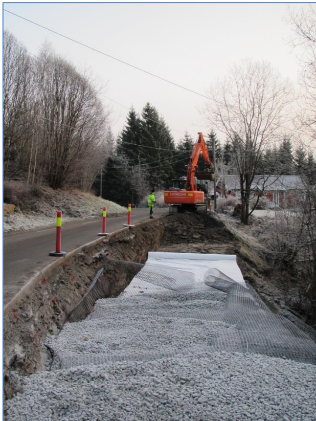
Figure 4: Foamglass is delivered. levert. Notice the geotextiles at the lower background in the picture. This slope is located on highway 120 north of Tomter, Østfold [14] .
