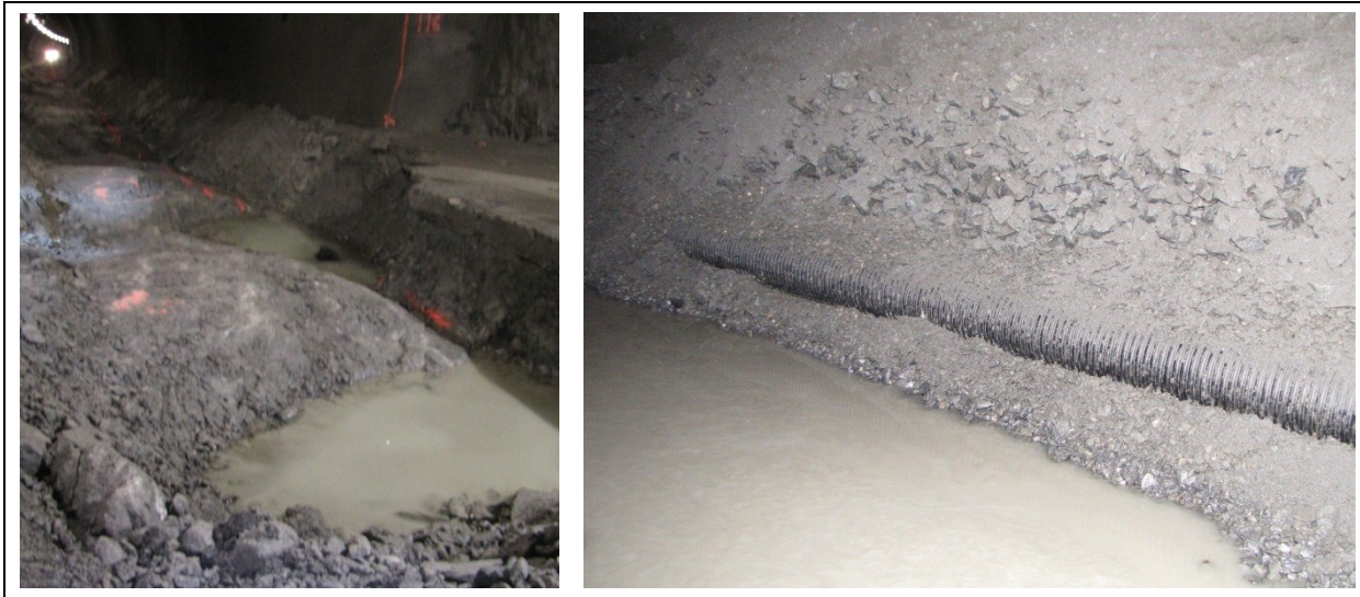
Figure 6: Undrained depressions in the rock-formation bed and shallow drainage pipe.
