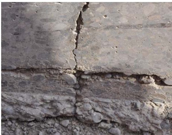
Figure 2: Eroded surface of CTB beside joint of the concrete pavement (longitudinal section)
