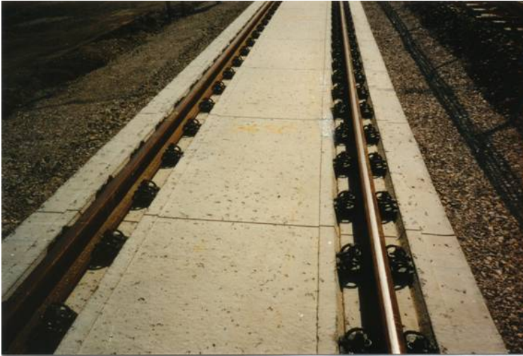
Figure 5: Ballastless track with discrete rail seats on a continuously reinforced concrete pavement (CRCP) with dummy joints to control transversal cracking.
