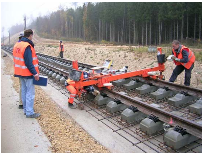
Figure 4: Track adjustment preparing for continuously reinforced concrete pavement (CRCP) on a cement treated base layer (CTB).
