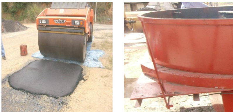
Figure 5. Aspect of the recycled mix compacted and leveraged from the device of mass discard.
