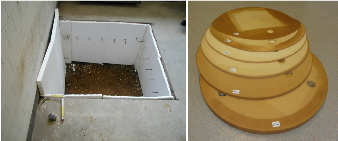
Figure 6: Decoupled formwork for concrete block (left) and rubber mats for calibration (right)
