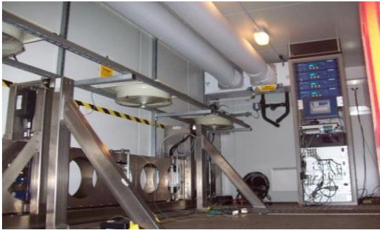
Figure 6a: Measurement beam after air conditioning fitted
