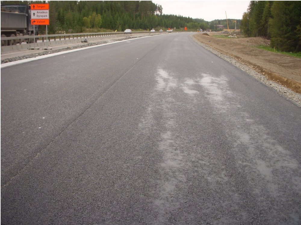
Figure 5: Pavement section fat areas
