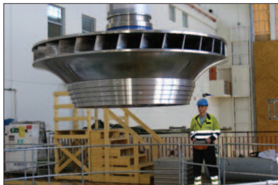
(d) The old runner being taken out, and the new one on its way in, at Hol 1. Photo: ECO Vannkraft.
