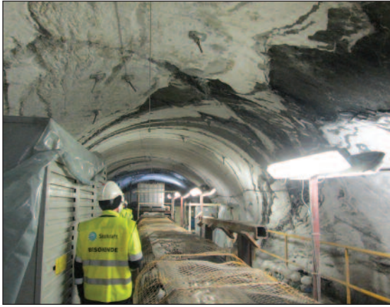
(h) The 7.2 m-diameter tunnel driven by TBM at Røssåga. Photo: Leif Lia.
