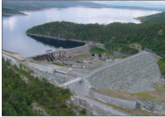
(j) Møsvatnet dam before demolition of the existing concrete dam. Photo: Øst-Telemarkens Brukseierforening.
